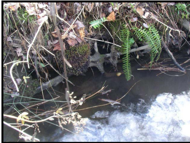
Figure 5—Typical Bank Scour
