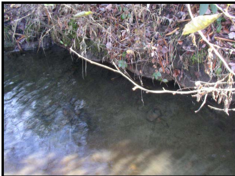
Figure 4—Typical Bank Scour
