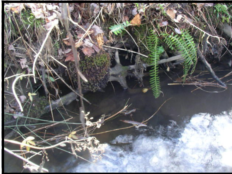
Figure 5—Typical Bank Scour (November 13, 2007)
