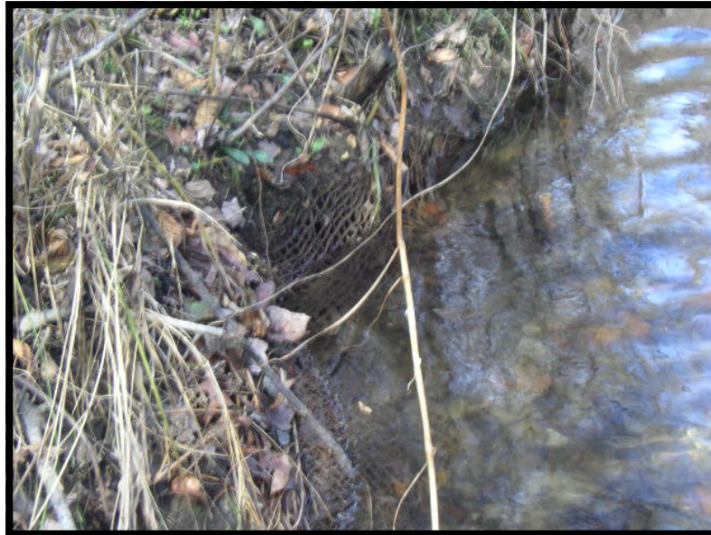
Figure 3— Typical Bank Scour (November 13, 2007)
