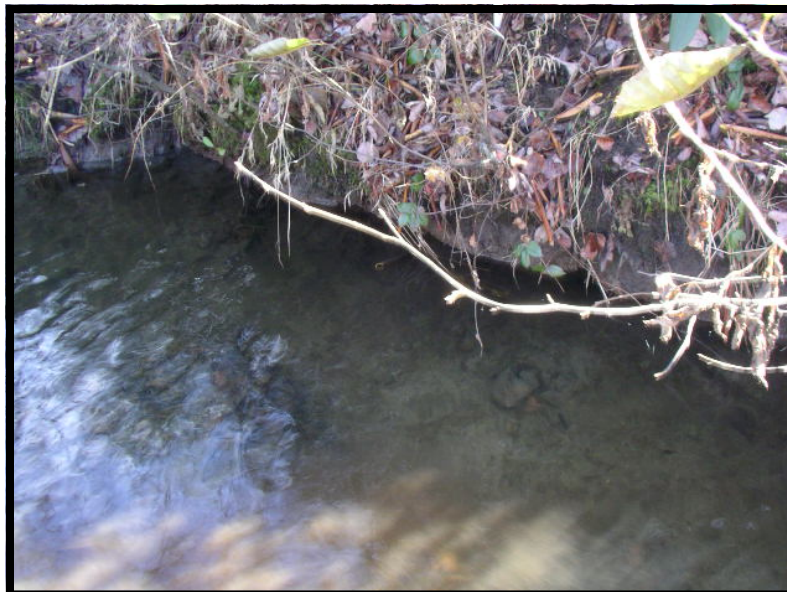
Figure 4— Typical Bank Scour (November 13, 2007)
