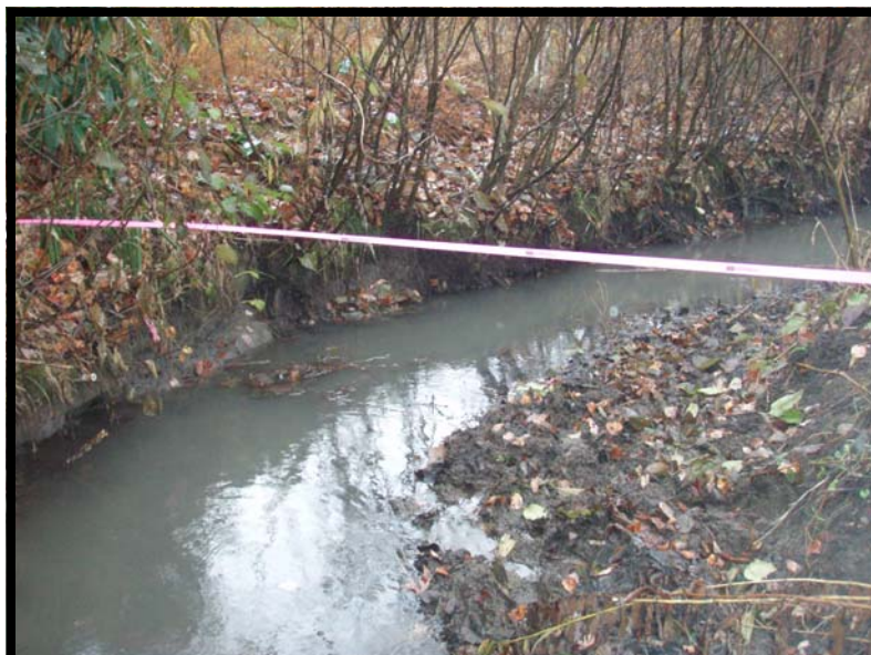
Figure 6—Typical Bank Scour (November 13, 2007)
