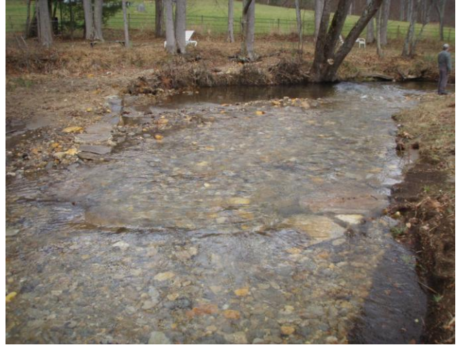
Aggradation and bar formation in meander below J-hook after flood event, 5 December 2012.
