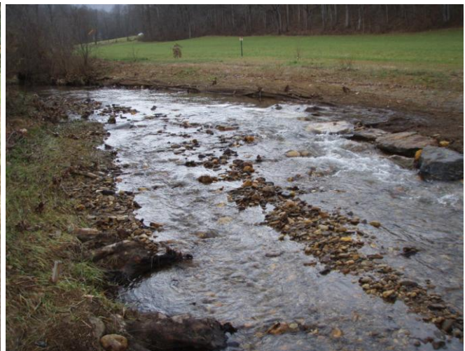
Aggradation and bar formation in below J-hook after flood event, 5 December 2012.
