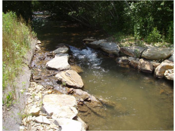
Rock vane after flood damage, sta. 1+50, 5 December 2012.
