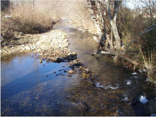
Bed aggradation and transverse bar, sta. 9+50 to 10+00, facing downstream, 22 January 2009.
