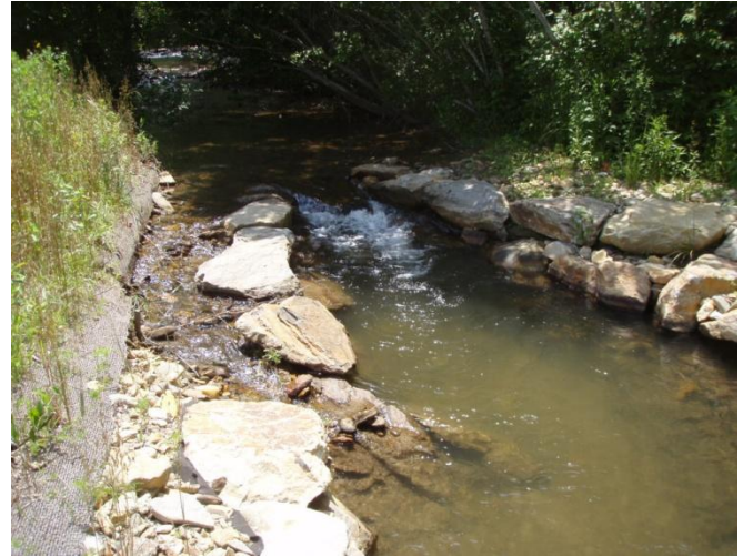
Rock vane after flood damage, sta. 1+50, facing upstream, 14 June 2012.
