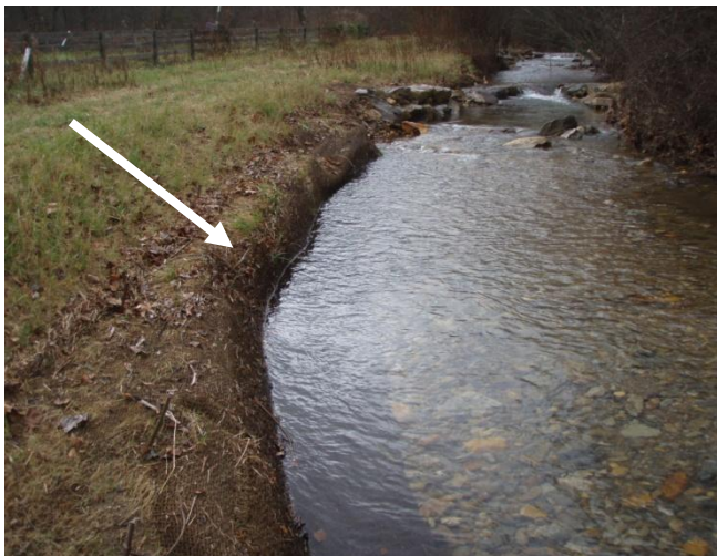
Right channel bank instability after flood damage, sta. 1+75 to 2+25, facing upstream, 5 December 2011.
