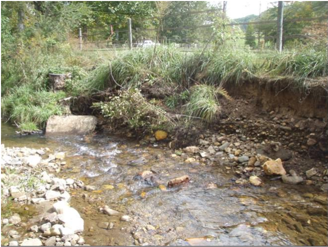
Right bank erosion, sta. 5+50, pre-construction, 30 September 2008.
