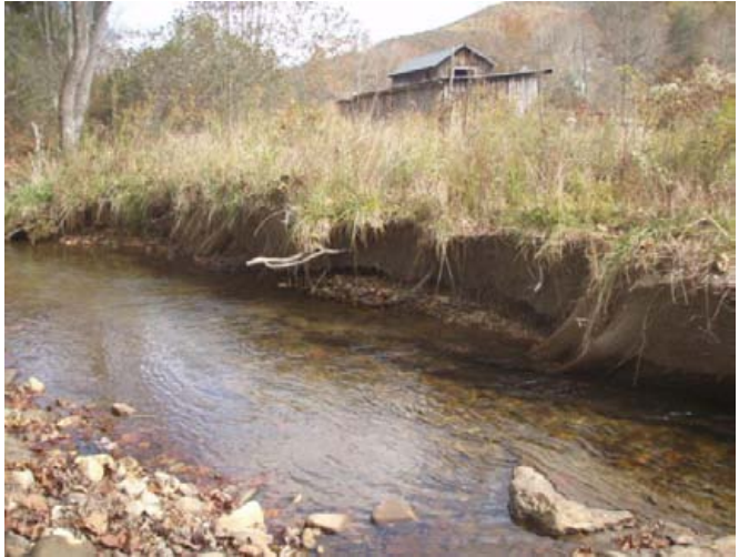
Right channel bank condition after 5 May 2013 flood, sta. 1+75 to 2+25, facing downstream, 29 October 2013.
