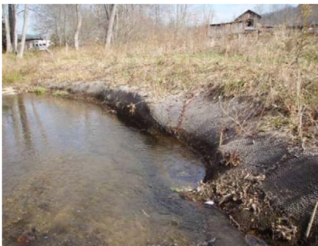
Right channel bank instability, sta. 1+75 to 2+25, facing downstream, 20 November 2012.
