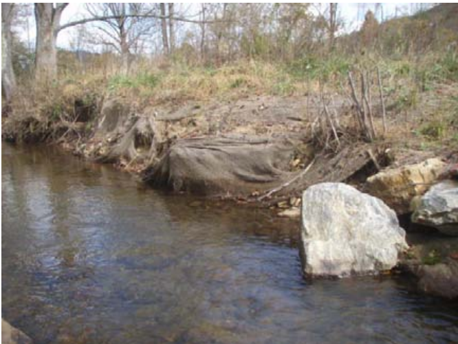
Right bank scour and erosion, sta. 6+25, facing downstream, occurred during the 5 May 2013 flood event, 29 October 2013.
