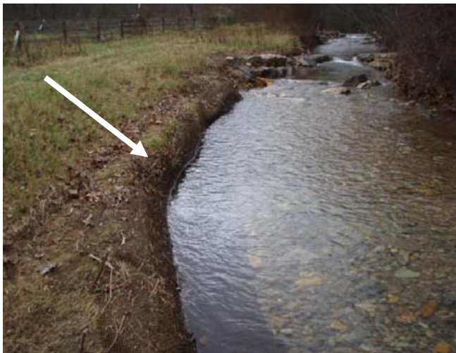
Right channel bank instability after flood damage, sta. 1+75 to 2+25, facing upstream, 5 December 2011.
