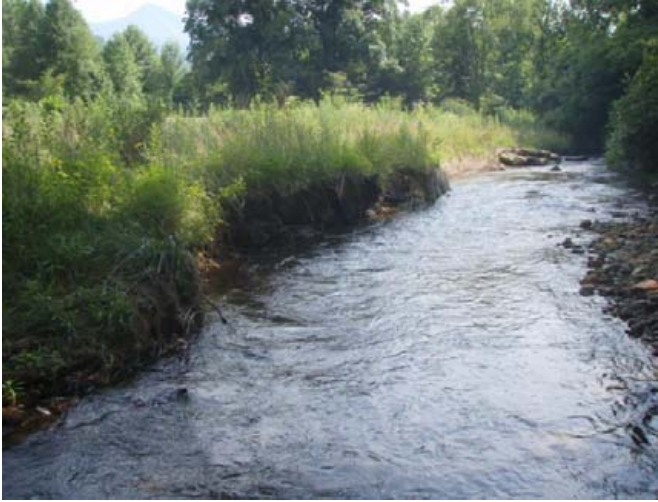
Right channel bank condition after 5 May 2013 flood, sta. 1+75 to 2+25 facing upstream, 18 July 2013.
