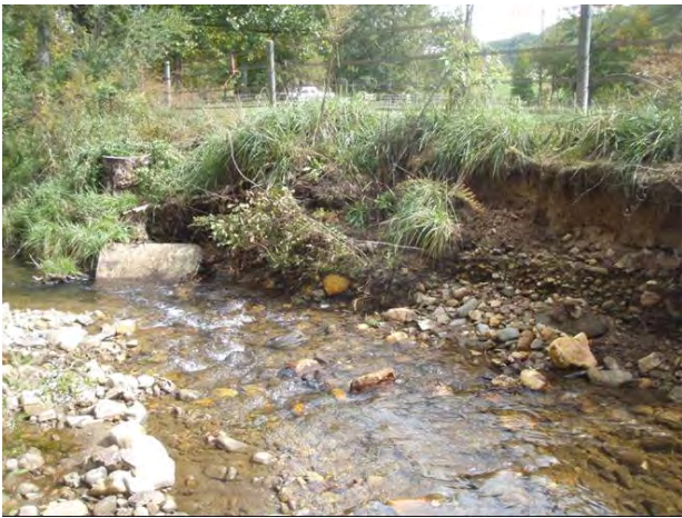
Right bank erosion, sta. 5+50, pre-construction, 30 September 2008.
