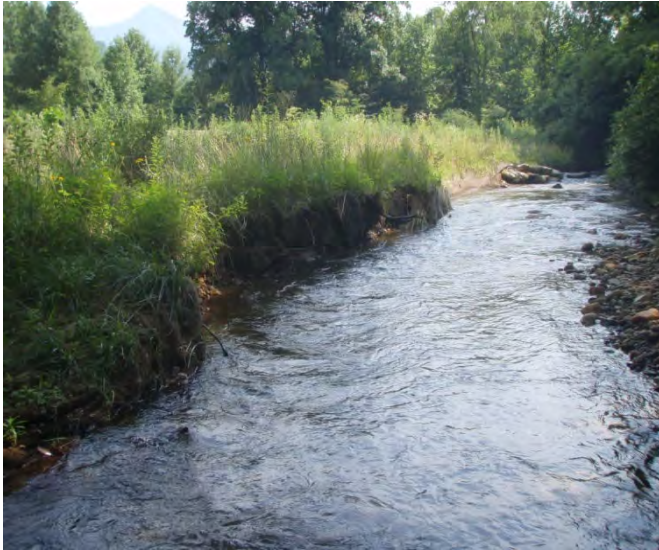
Right channel bank condition after 5 May 2013 flood, sta. 1+75 to 2+25 facing upstream, 18 July 2013.
