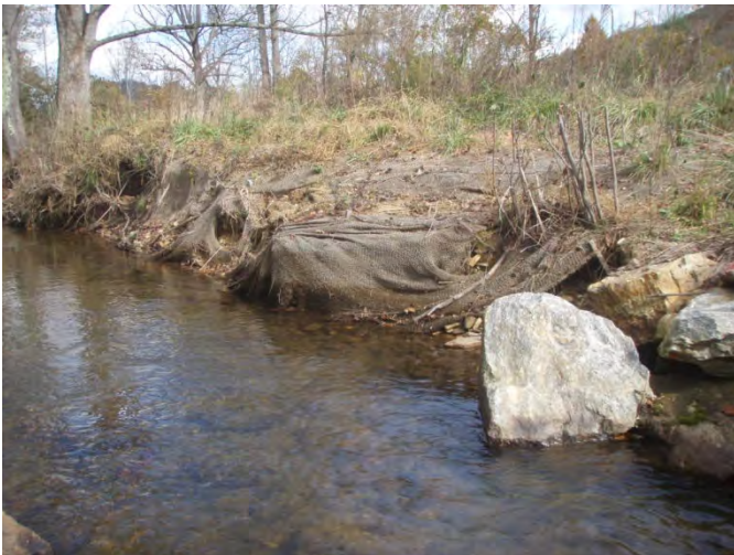
Right bank scour and erosion, sta. 6+25, facing downstream, occurred during the 5 May 2013 flood event, 29 October 2013.
