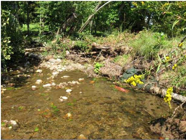
Channel blockage, sta.2+50, facing downstream, pre-construction, 30 September 2008.
