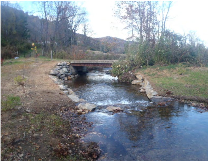
PA-7 station 12+75 facing downstream was repaired and is no longer considered a problem 28 October 2014
