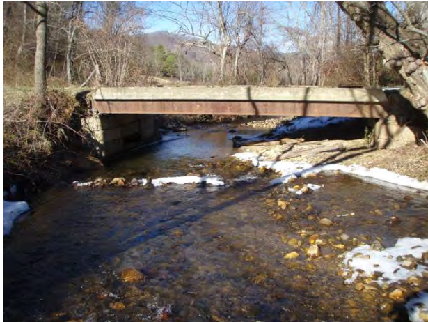
Driveway bridge at lower end of Bura/Roberson properties, sta. 12+50, facing downstream, 22 January 2009.
