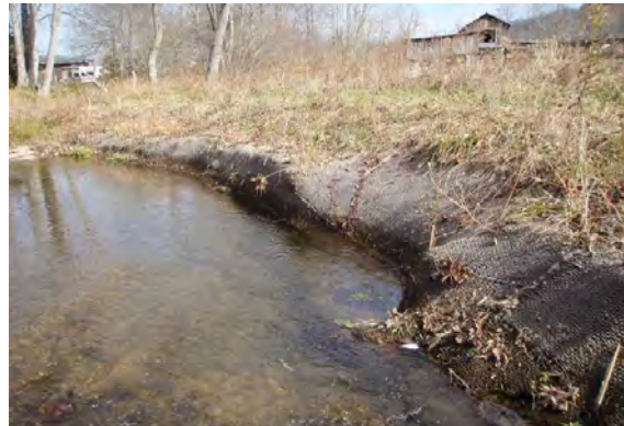
Right channel bank instability, sta. 1+75 to 2+25, facing downstream, 20 November 2012.
