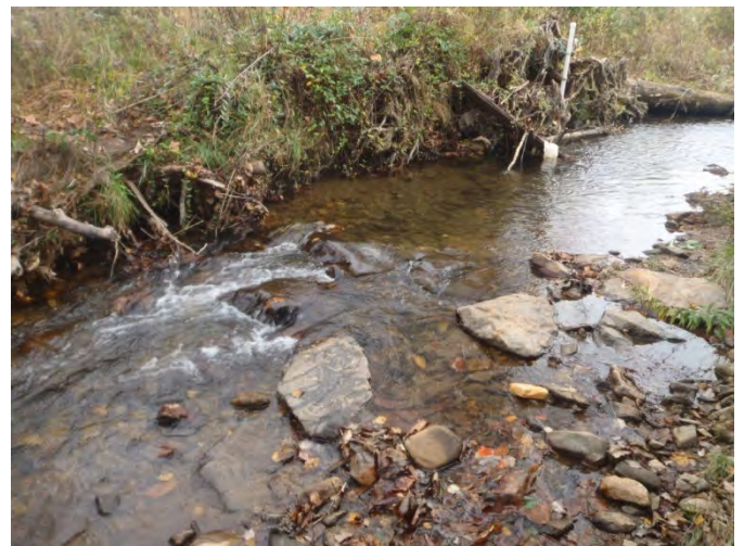
Right bank scour and erosion, sta 6+25 to 6+50 facing upstream, 28 October 2014
