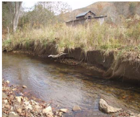
Right channel bank condition after 5 May 2013 flood, sta. 1+75 to 2+25, facing downstream, 29 October 2013.
