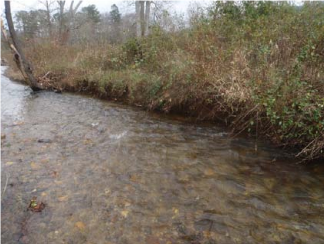
Right bank erosion due to high flow events, sta. 5+05 to 6+10 facing downstream, 17 November 2015.
