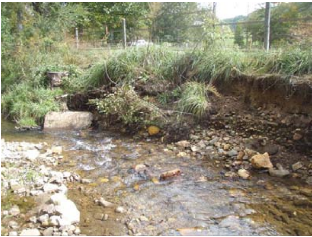
Right bank erosion, sta. 5+50, pre-construction, 30 September 2008.
