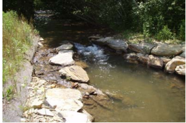
Rock vane after flood damage, sta. 1+50, facing upstream, 14 June 2012.
