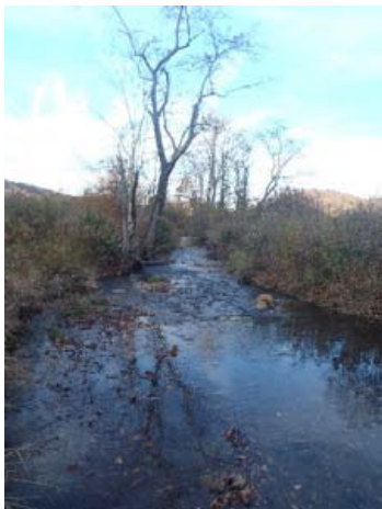
Log vane, root wads, and bank shaping, sta. 2+25 to 3+50, facing downstream, 12 Nov 2014.
