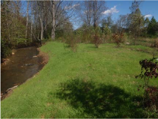
Right bank repairs performed summer 2015, sta. 6+25, facing downstream, 14 October 2015. No longer considered a problem during MY4 (2015) field surveys.
