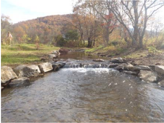
PA-7 station 12+75 facing upstream was repaired and is no longer considered a problem 28 October 2014
