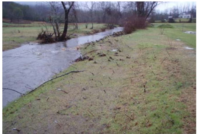
Log vane, root wads, and bank shaping, sta. 2+25 to 3+50, facing downstream, 7 December 2011.
