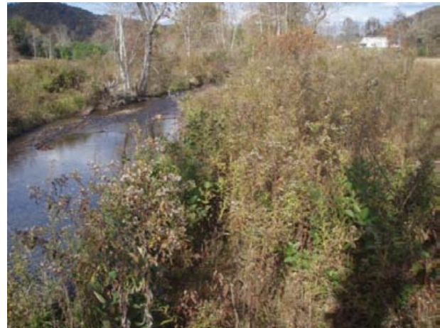
Log vane, root wads, and bank shaping, sta. 2+25 to 3+50, facing downstream, 29 October 2013.
