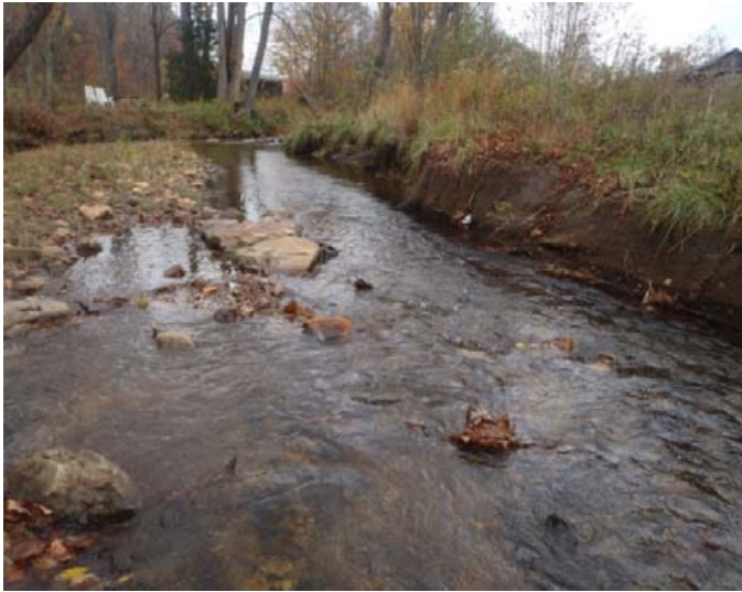
Aggradation below J-hook sta 2+50 facing downstream 28 October 2014
