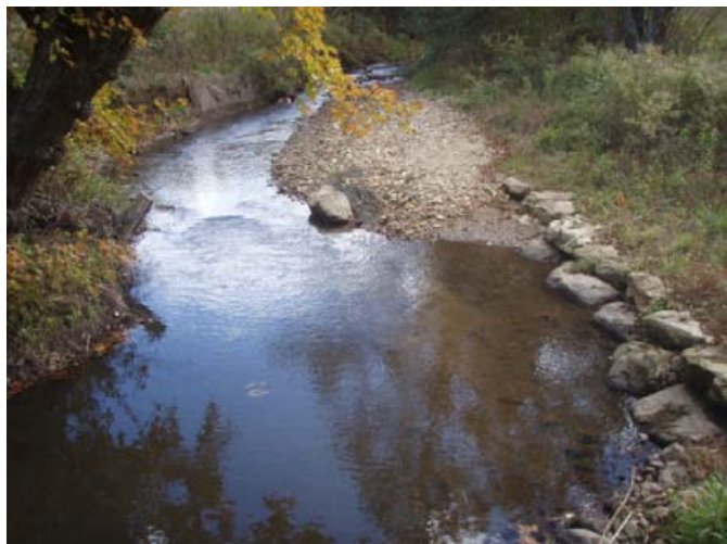
J-hook after 5 May 2013 flood event, aggradation above J-hook and scour pool below, 29 October 2013.
