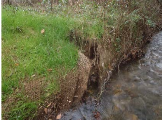
Right bank erosion due to high flow events, sta. 5+05 to 6+10 facing upstream, 17 November 2015
