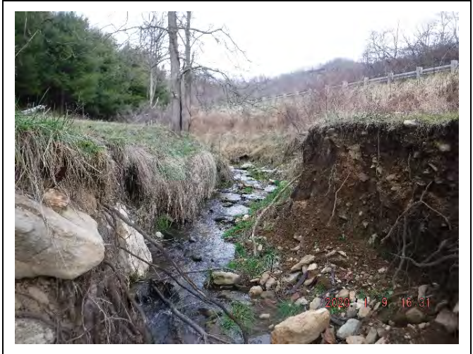
UT1-R4, culverted crossing wash-out upstream (Jan. 2020)
