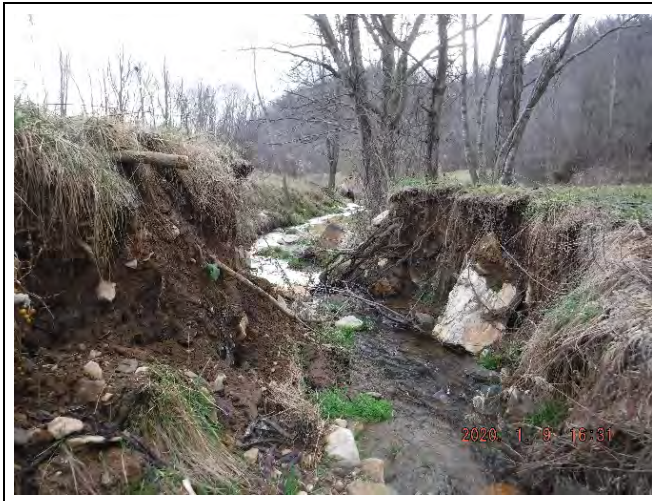
UT1-R4, culverted crossing wash-out downstream (Jan. 2020)
