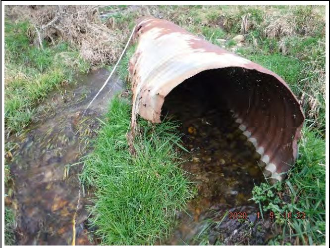
UT1-R4, downstream at dislodged culvert (Jan 2020)
