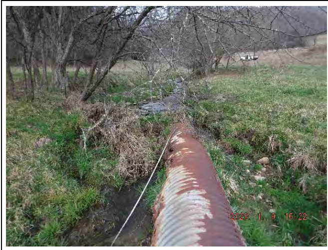
UT1-R4, upstream at dislodged culvert (Jan. 2020)
