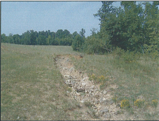
Photo 5. Facing southwest along the emergency spillway situated immediately outside of the conservation easement area.
