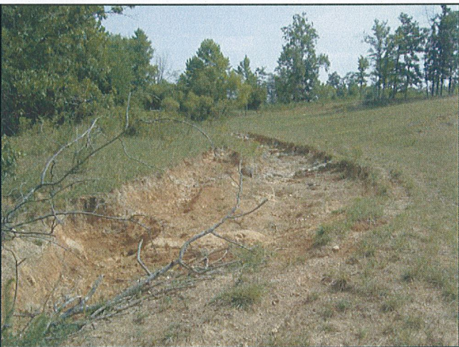
Photo 6. Facing northeast along the emergency spillway situated immediately outside of the conservation easement area.
