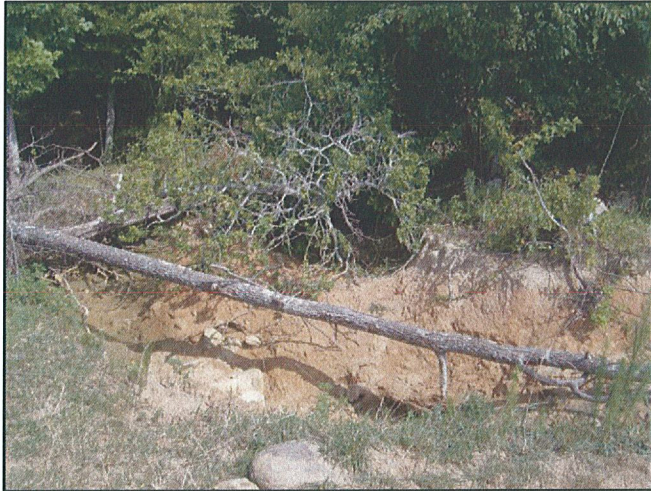
Photo 7. Facing northwest at the scour associated with the emergency spillway within the conservation easement area.
