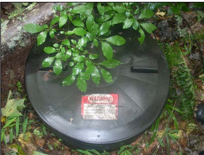
Potable water reservoir located in the conservation easement.
