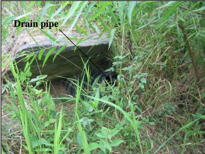
Outlet structure (black pipe below the rock) is well above the water line.
