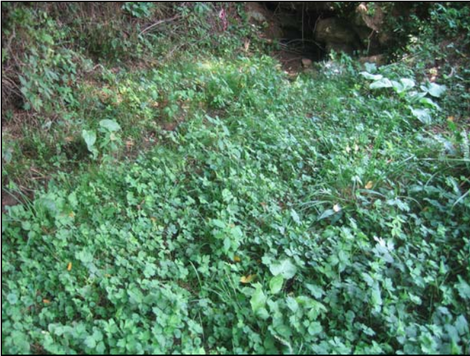
Surface water disappears from channel just before entering the culvert under Sweet Hollow Road.
