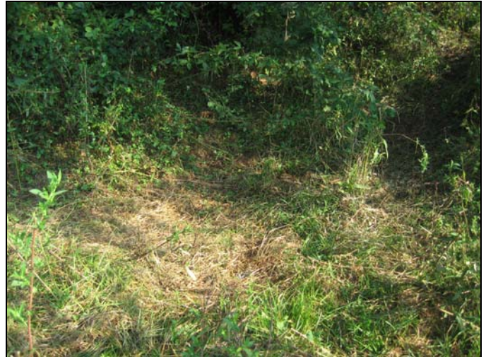
Base of the dam below Sweet Hollow Road, showing the absence of a stream channel.
