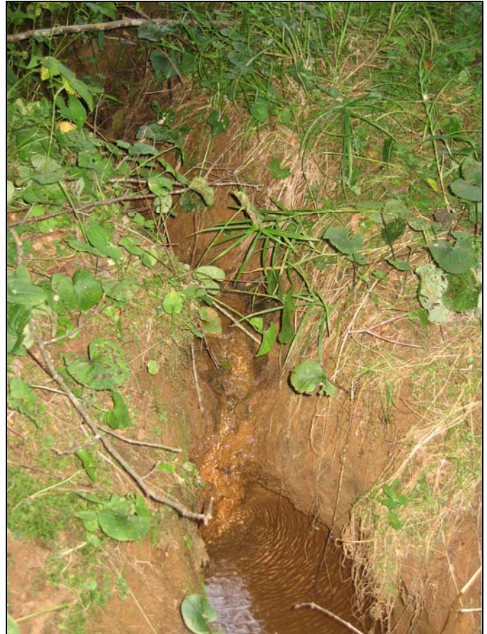
Headcut below perennial origin of Tributary 1.
