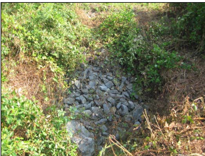
Riprap on downstream side of dam – presumed to be location of pipe outlet.
