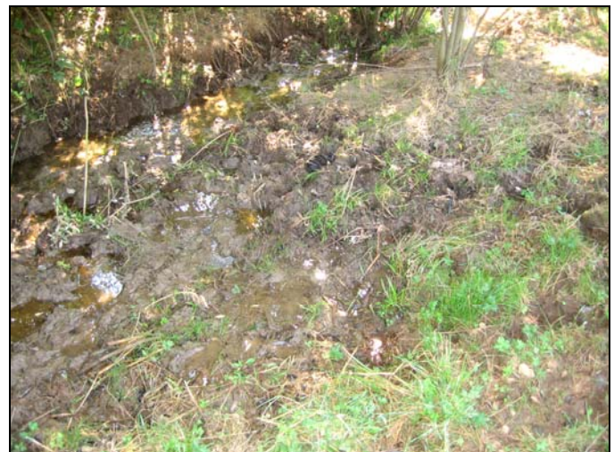
A groundwater seep flows into the channel just above the last proposed crossing near the barn.
