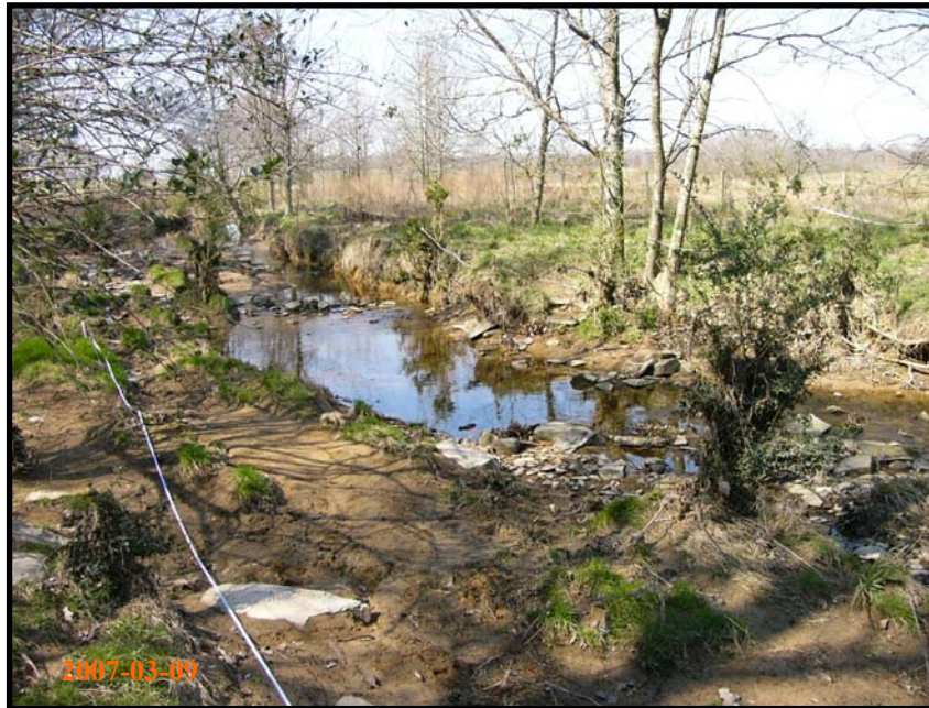
Northern UT where the channel has incised to bedrock and high shear stress is being placed on banks.
