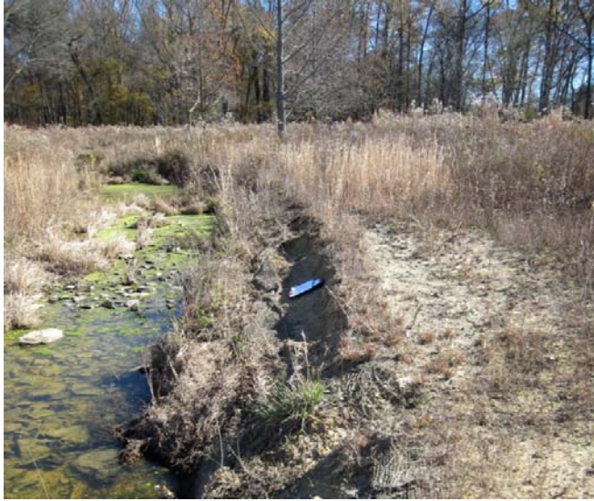
5. Bank Scour (Sta. 29+15) - Northern UT
