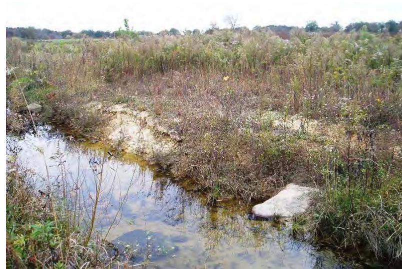
8. N-sta-3470.LB Erosion.Thin Herb Cover, No Woody
