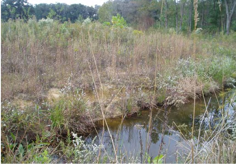
1. N-sta-3450.LB Erosion.Oct 2013. Thin veg cover, no woody.
