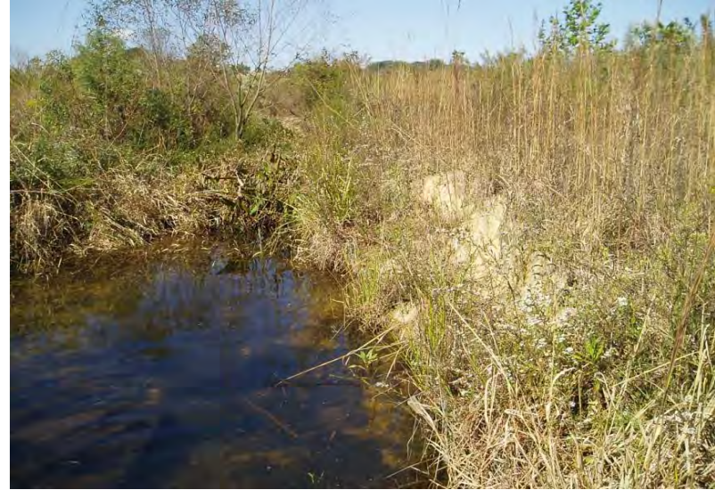
2. N-sta-3450.LB Erosion.Oct 2013. Thin veg cover, no woody.
