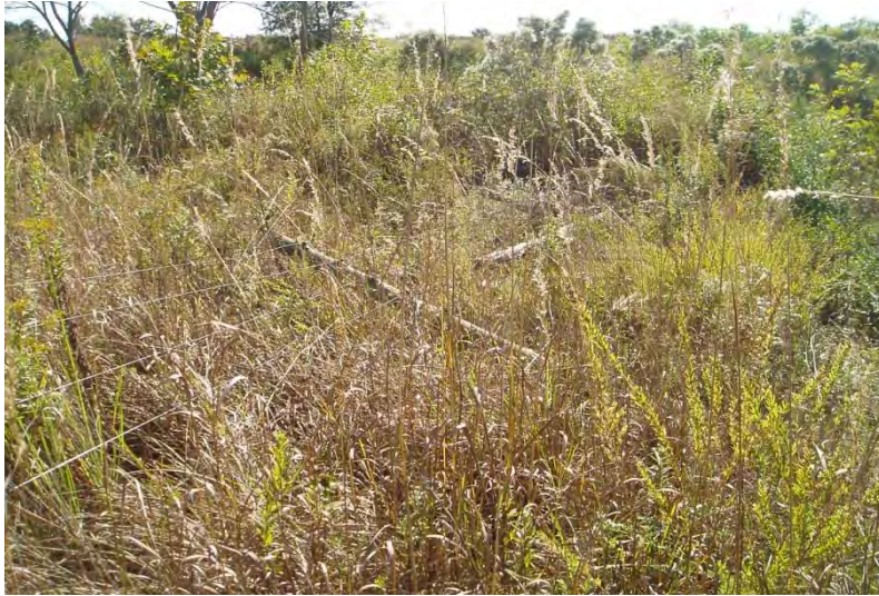
9. N-sta-1930.LB. Oct.2013. Fence collapse at cattle crossing
