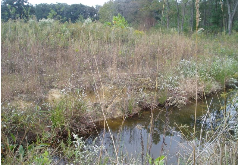
1. N-sta-3450.LB Erosion.Oct 2014. Thin veg cover, no woody.
