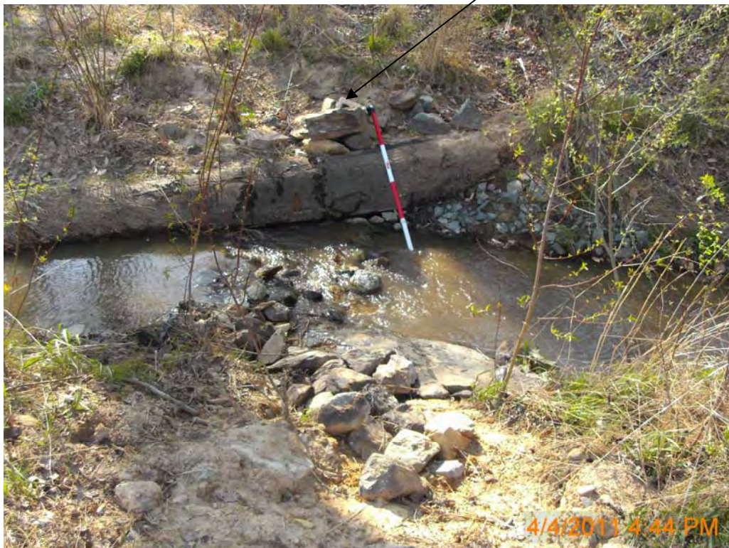
Photo taken from right bank looking at the log structure (note cinder block on left bank)
