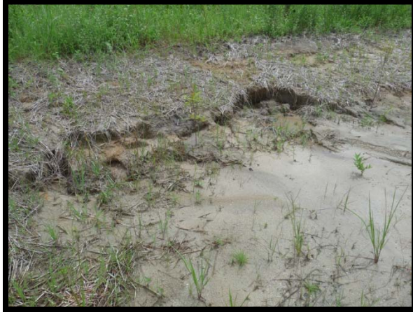
3.17 Bare area on terrace slope
