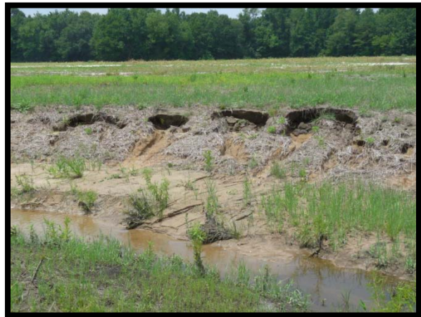
3.20 Wash areas on terrace slope
