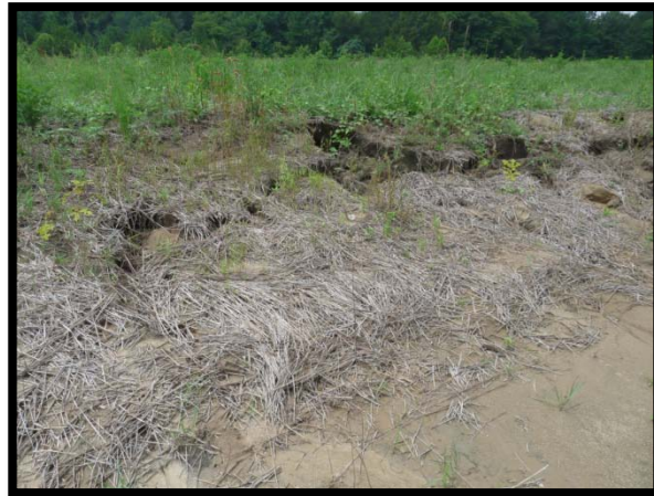
3.16 Bare area on terrace slope
