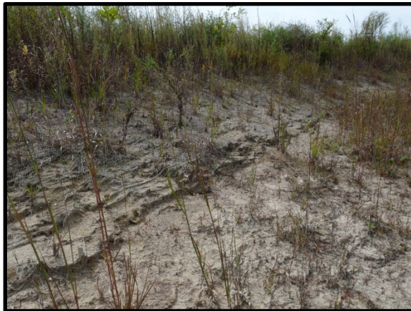
3.19 Minor wash on terrace slope near station 35+00.
