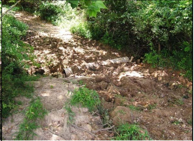
Inadequate culvert crossing on UT1-3
