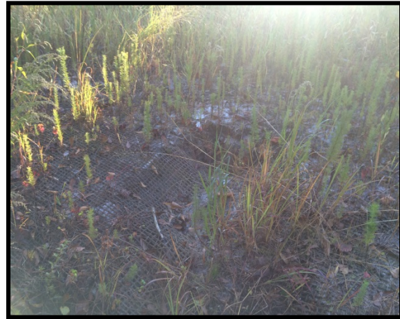
3.12 Minor gully near STA 19+00
