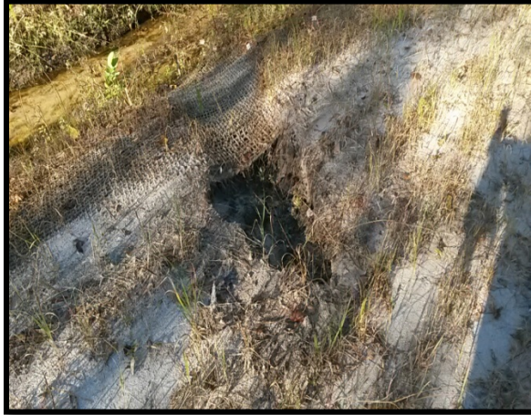
3.13 Gully on left bank at STA 34+00
