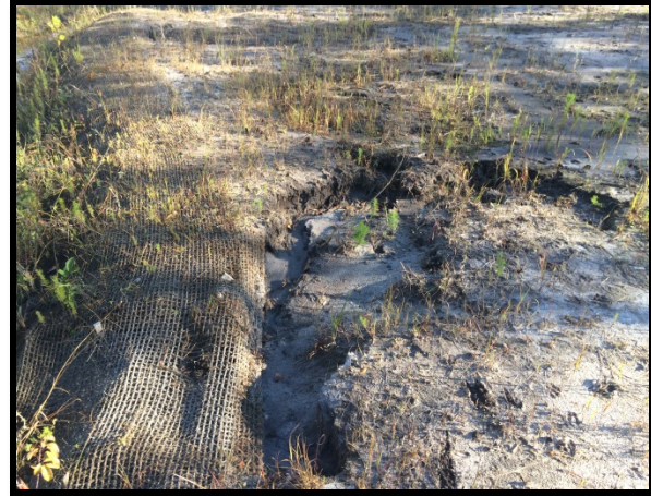
3.14 Gully on right bank at STA 34+50
