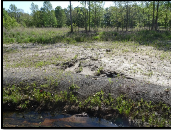
3.13 Gully on left bank at STA 34+00
