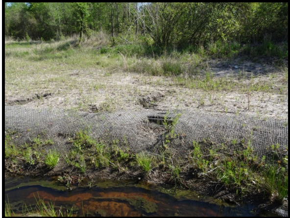
3.14 Gully on right bank at STA 34+50
