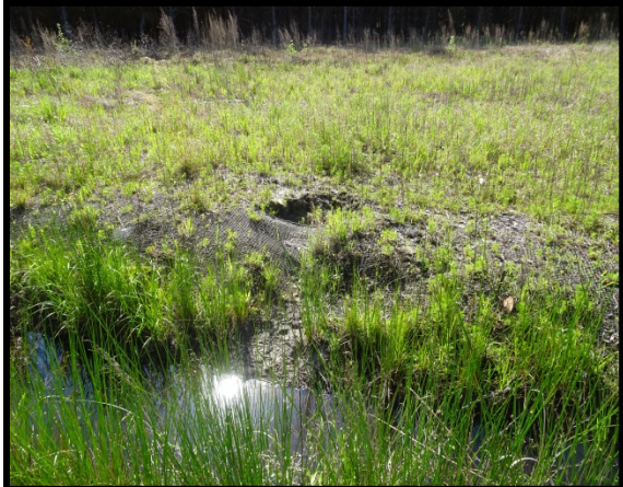
3.12 Minor gully near STA 19+00
