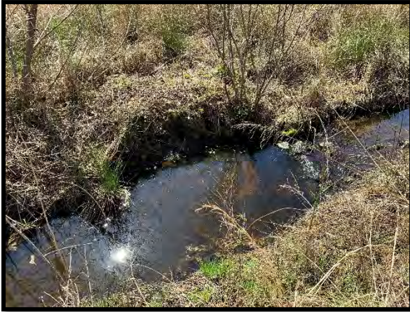
3.11 Minor bank erosion near STA 30+00
