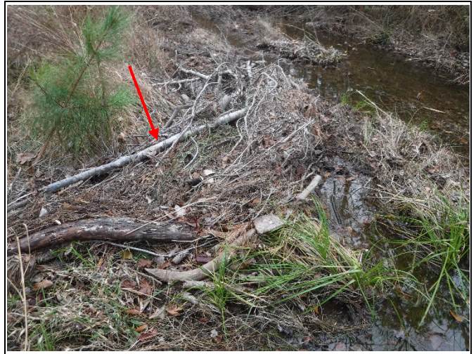
Debris and wrack lines in the floodplain from overbank event on UT-1b (photo from 12/6/19)
