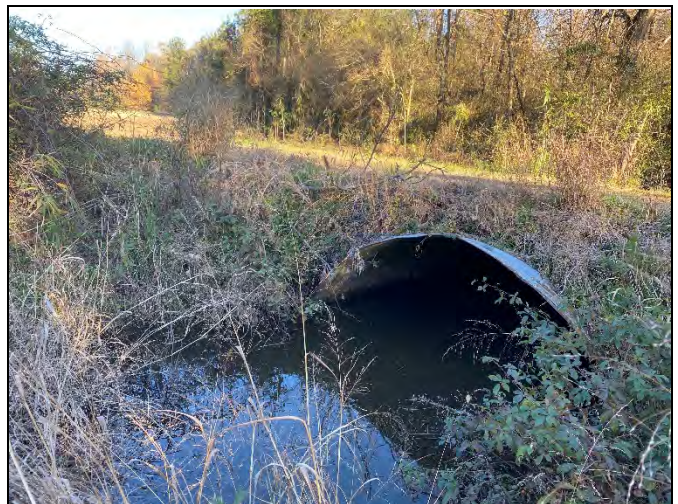
The culvert at the crossing at the bottom of the project (outside of easement).
