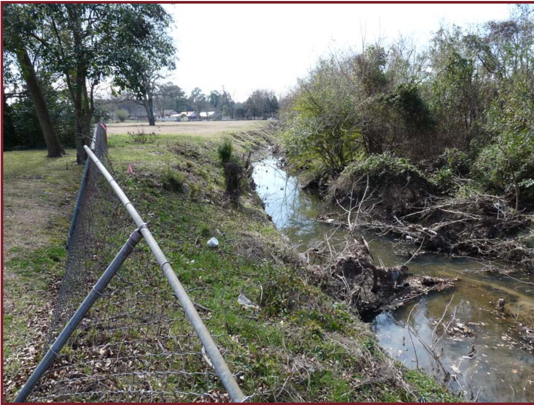
Photo 3 – Incised channel with eroding side slopes and undermined chain link fence
