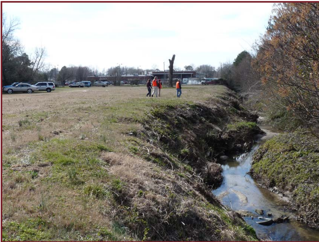
Photo 6 – Incised channel with steep and sloughing channel banks
