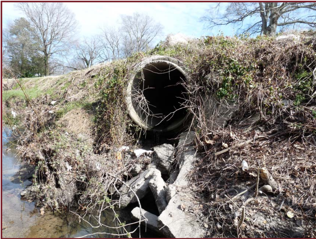
Photo 5 – Perched culvert with scrap concrete dissipator to prevent further erosion
