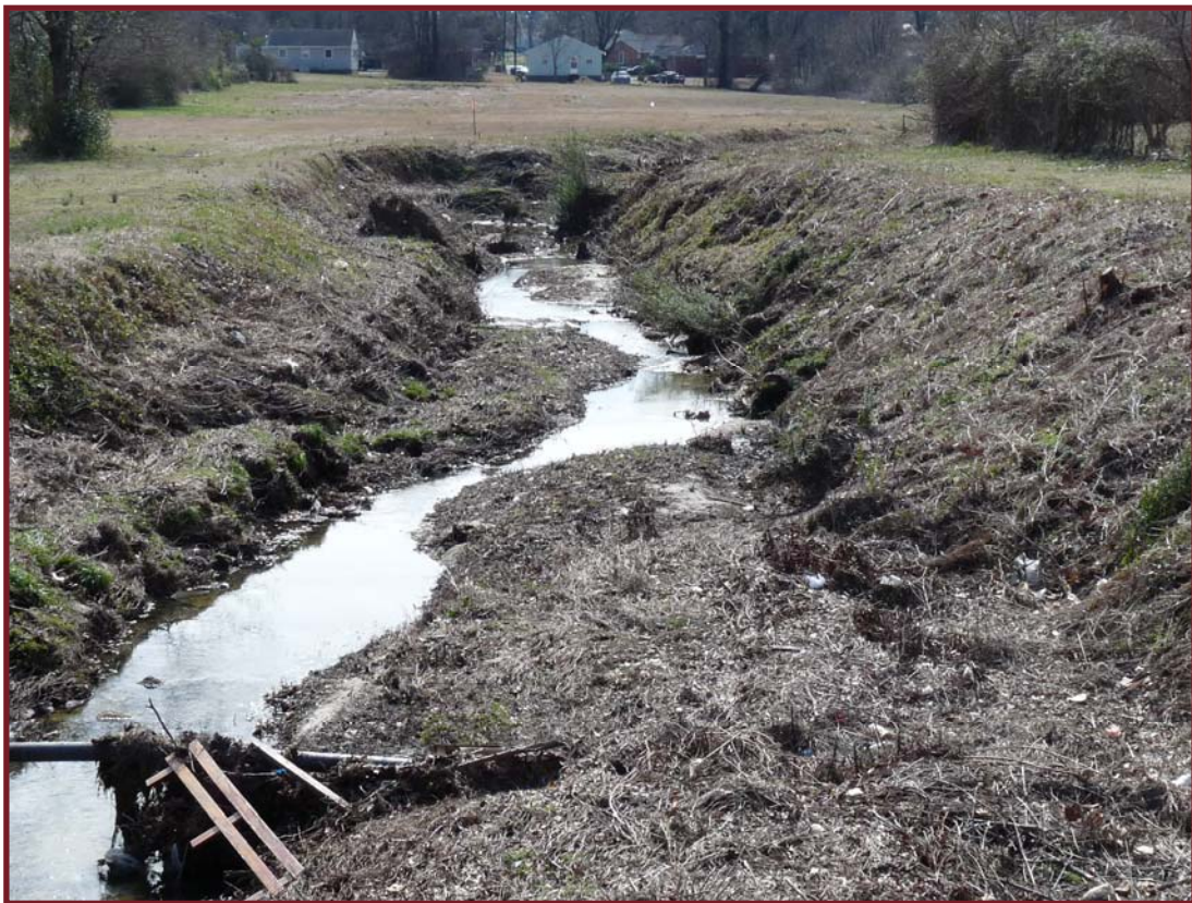
Photo 2 – Sewer line within incised channel, steep channel banks with erosion
