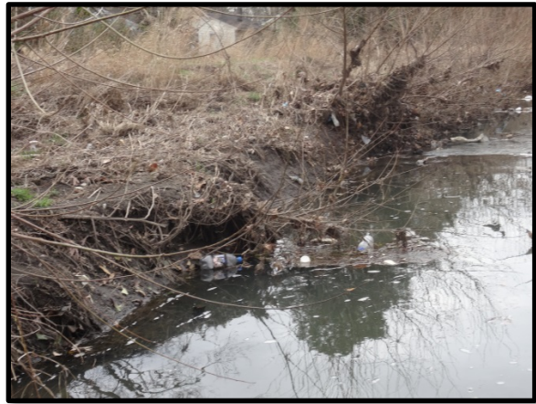
3.9 Minor Erosion Station 12+00
