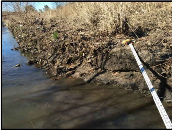
3.10 Moderate Erosion Station
