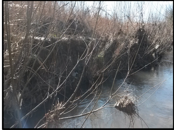
3.13 Moderate Erosion Station 30+00
