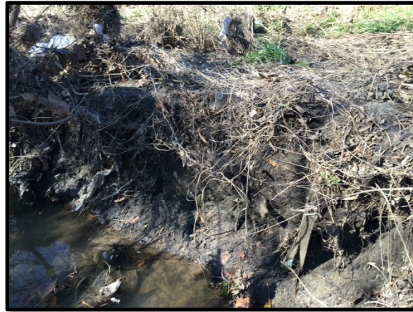
3.11 Moderate Erosion Station 14+50
