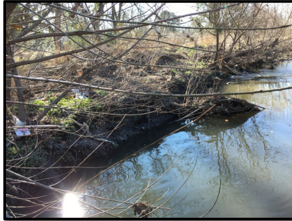
3.9 Minor Erosion Station 12+00
