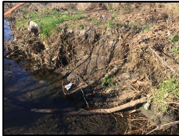
3.11 Moderate Erosion Station 14+50
