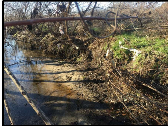
3.9 Minor Erosion Station 11+00
