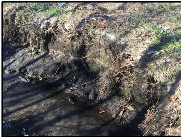
3.10 Moderate Erosion Station 13+00
