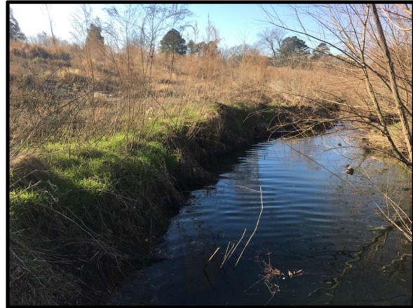
3.13 Minor Erosion Station 23+00
