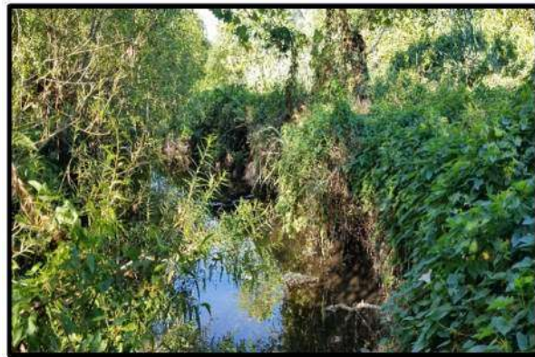
3.11 Moderate Erosion Station 14+00
