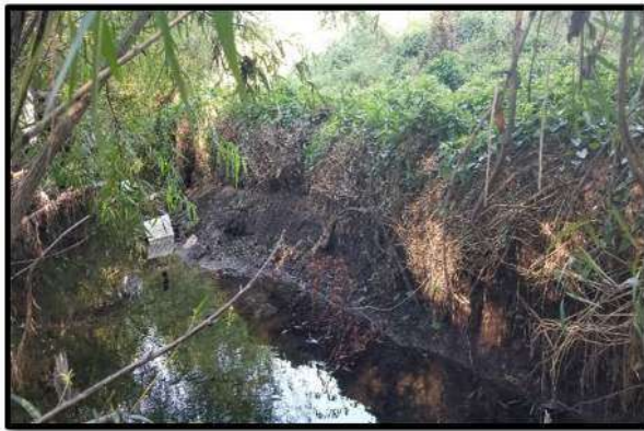
3.10 Minor Erosion Station 13+00
