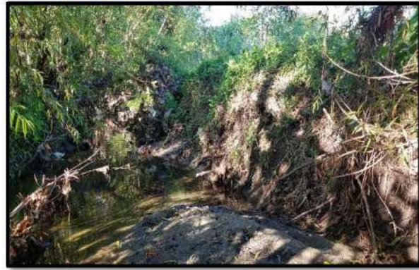
3.9 Minor Erosion Station 11+00
