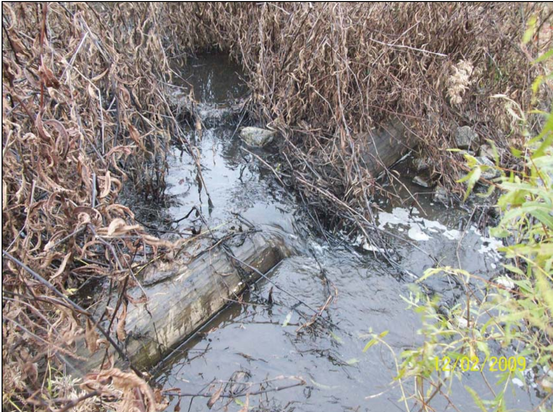
Maintenance Photo – 12/2/09 - MY 02 – Water flowing through notch in second log of grade transition.
