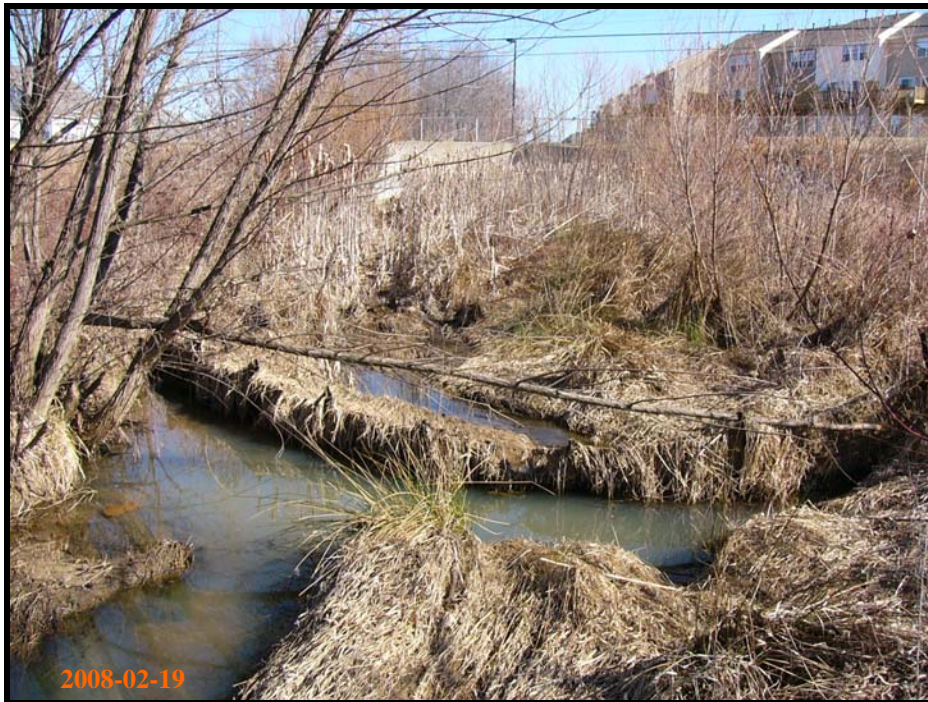
Silt fence traversing channel causing backwater through upstream culvert.
