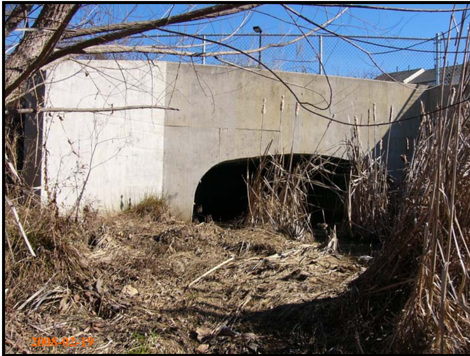
Silted in culvert at upstream end of Site.
