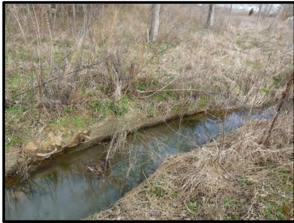
3.19 Eroded right bank near 14+50
