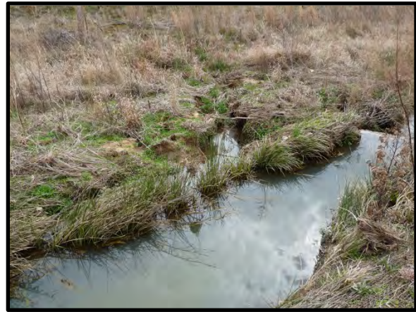
3.20 Eroded left bank near 20+90
