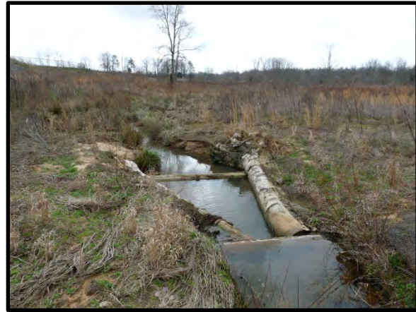
3.22 Double step log cross vane, notice water piping under second log step
