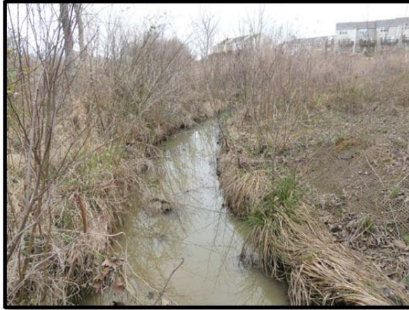
3.17 Minor bank erosion at Station 15+00 facing downstream
