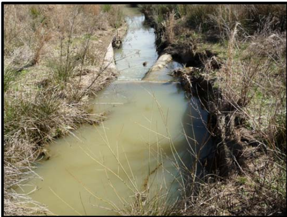
3.23 Eroded bank Station 35+80 facing downstream
