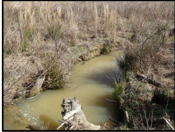
3.22 Moderate bank erosion at Station 34+25 facing downstream
