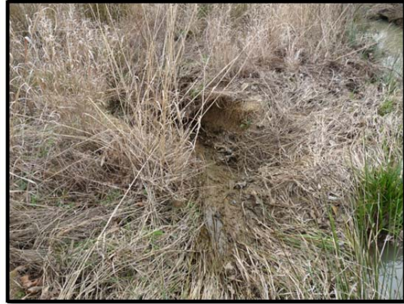
3.18 Minor bank erosion at Station 20+90 facing left bank
