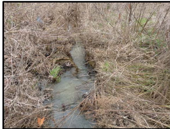
3.16 Small headcut at Station 14+20 facing downstream
