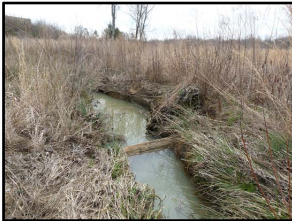
3.19 Erosion and piping at Station 20+90 facing downstream
