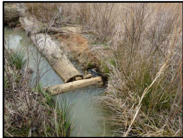
3.20 Piping of structure at Station 22+30 facing downstream
