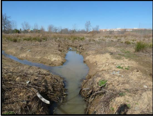
3.21 Beaver damage Station 33+30 facing upstream
