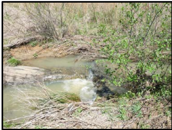
3.17 Major erosion near 22+50
