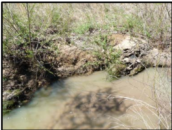
3.18 Major erosion below 35+00
