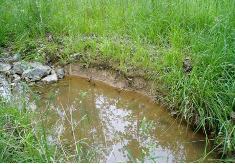
SP5 - Scour, Reach 2 (10/23/08)
