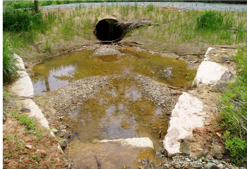
SP2 - Aggradation below Cross Vane, Reach 2 (10/23/08)
