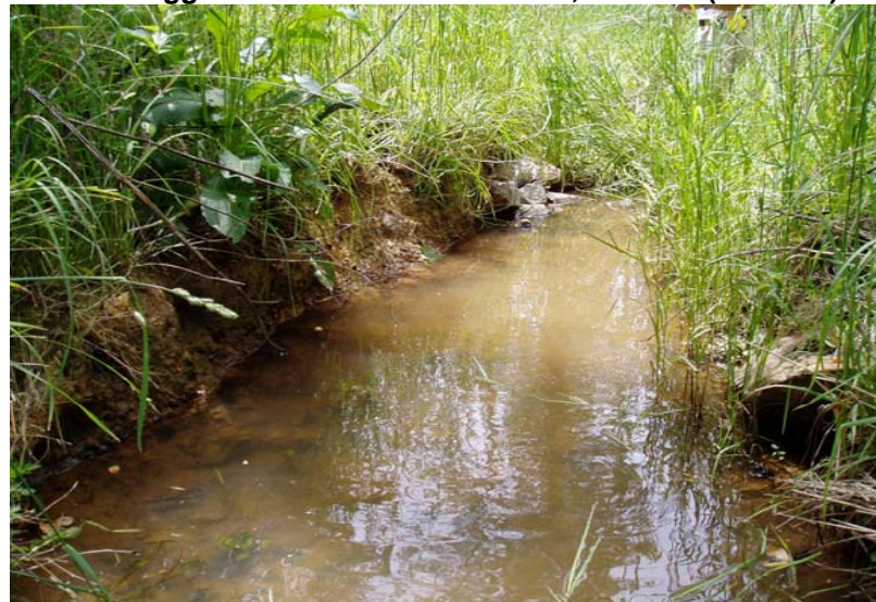
SP4 - Scour, Reach 2 (10/23/08)
