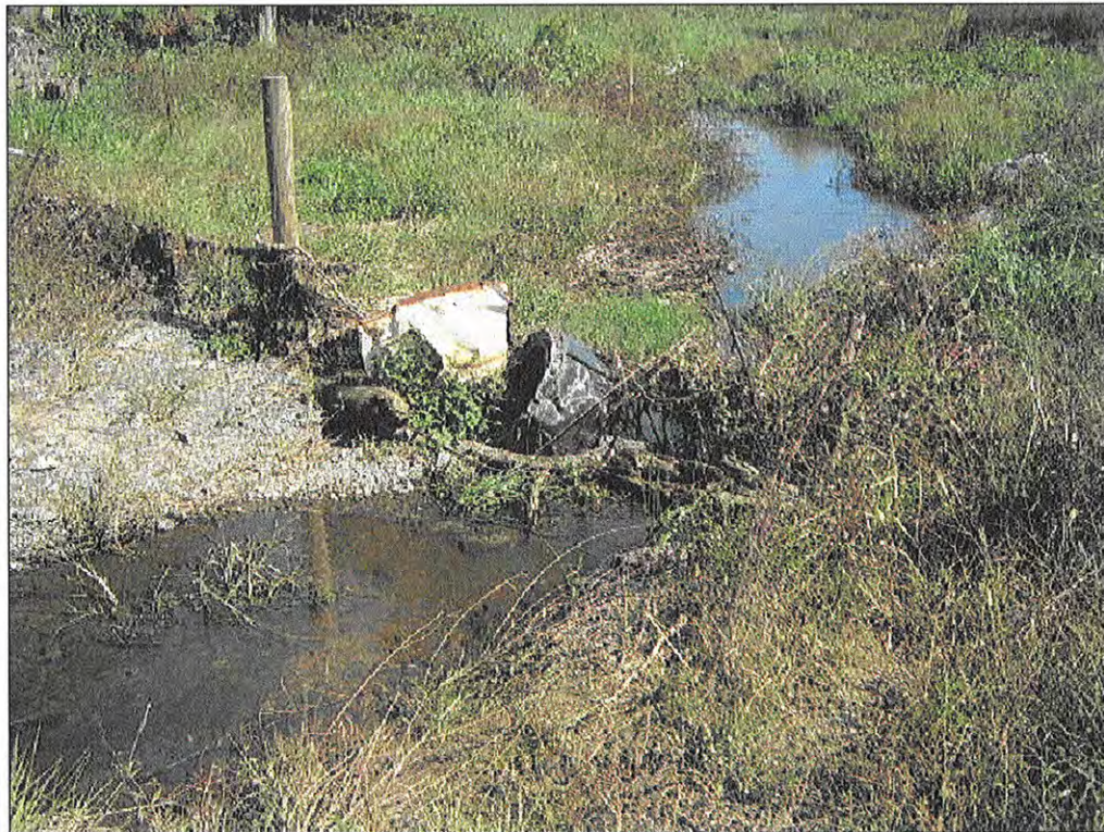
STREAM PROBLEM AREA 8. TRASH IN CHANNEL AT STATION 112+00.
