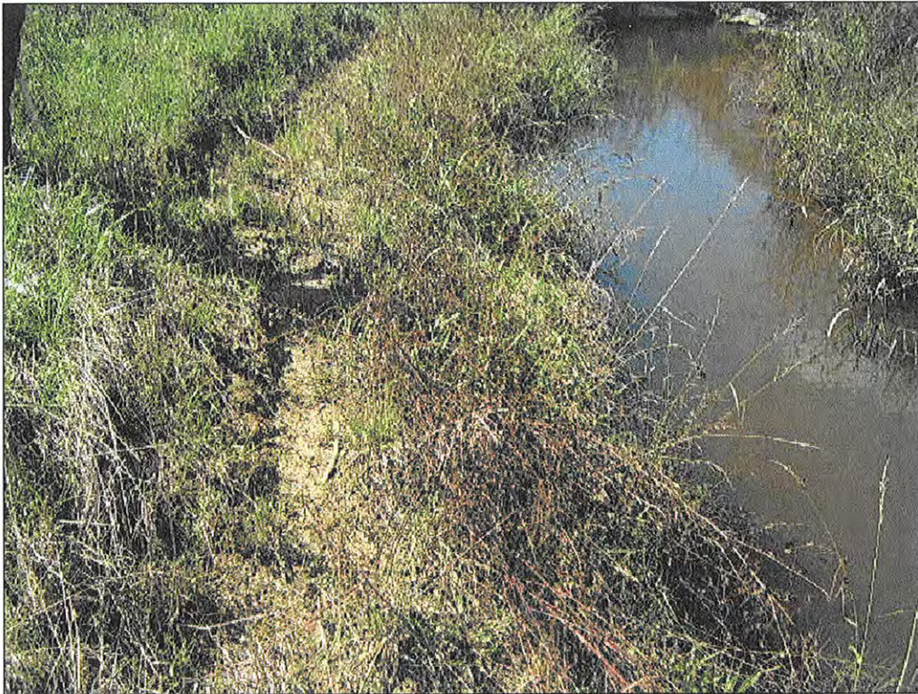
STREAM PROBLEM AREA 7. ERODING BANKS AT STATION 116+92 - 117+10.
