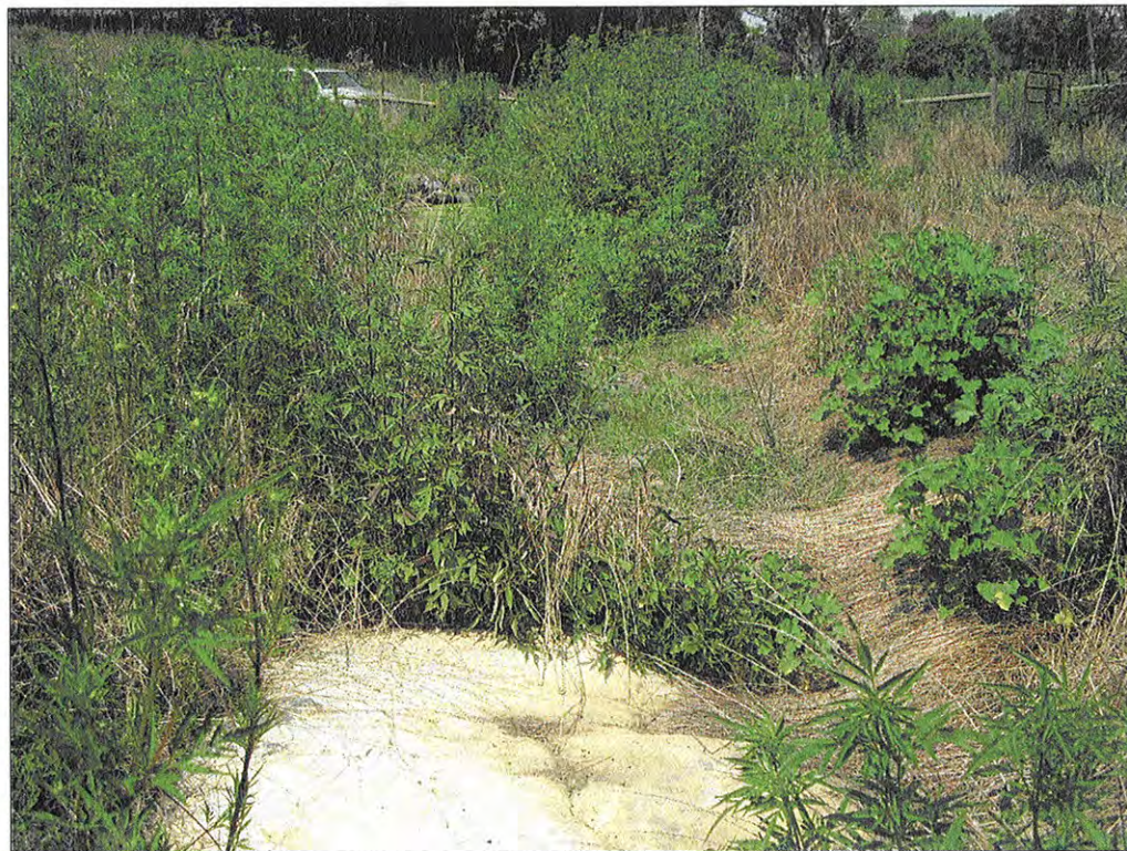
PHOTOGRAPH 24: CROSS VANE. STA: III+66.
