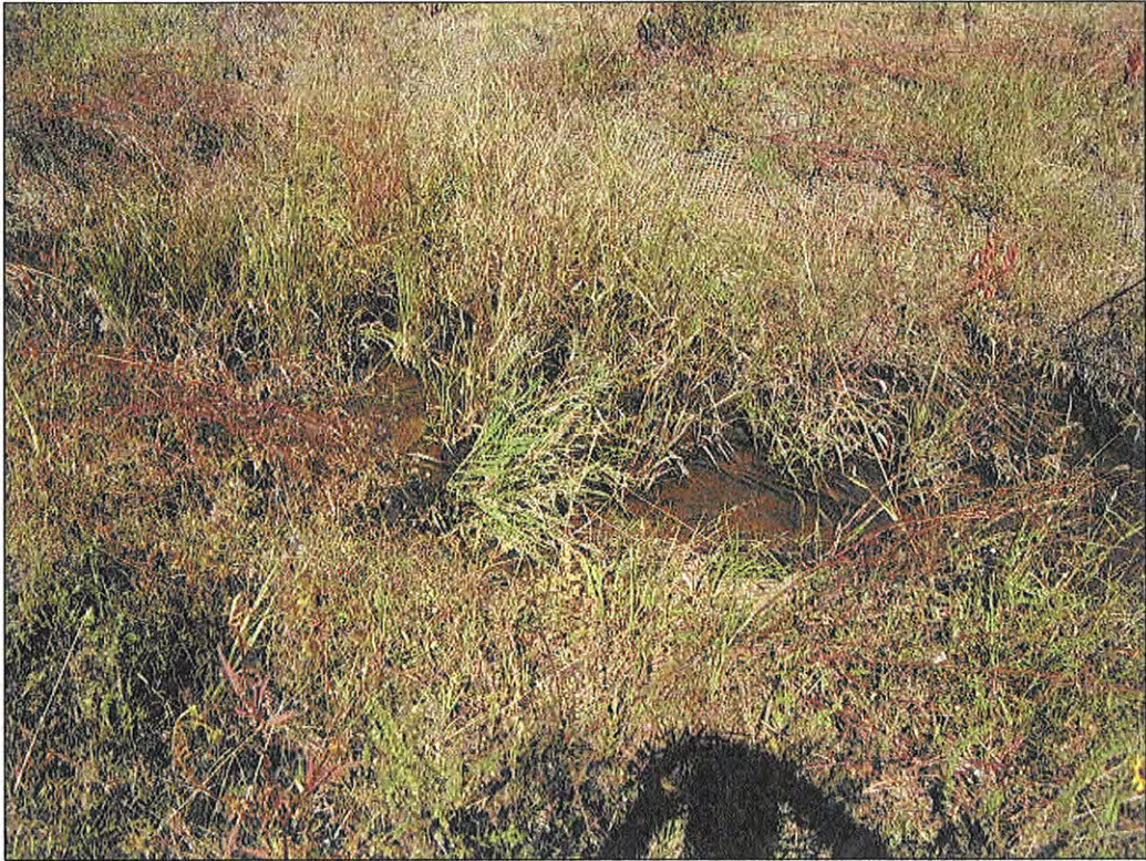
STREAM PROBLEM AREA 3: AGGRADATION AND VEGETATION IN CHANNEL INFLUENCING CHANNEL MORPHOLOGY AT STATION 118+25.
