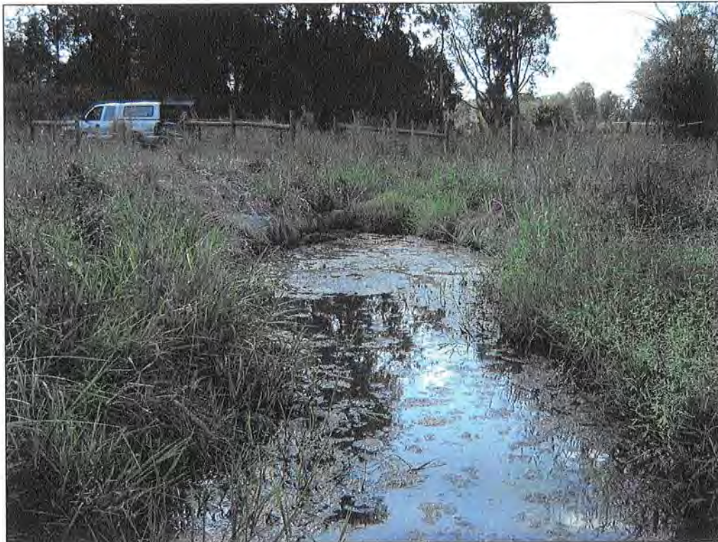
PHOTOGRAPH 24: CROSS VANE. STA: III+66.
