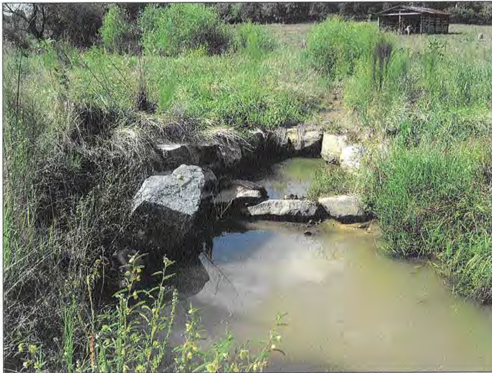
STREAM PROBLEM AREA 9. BOULDER COMING LOOSE AT "A" VANE STA: 116+29.
