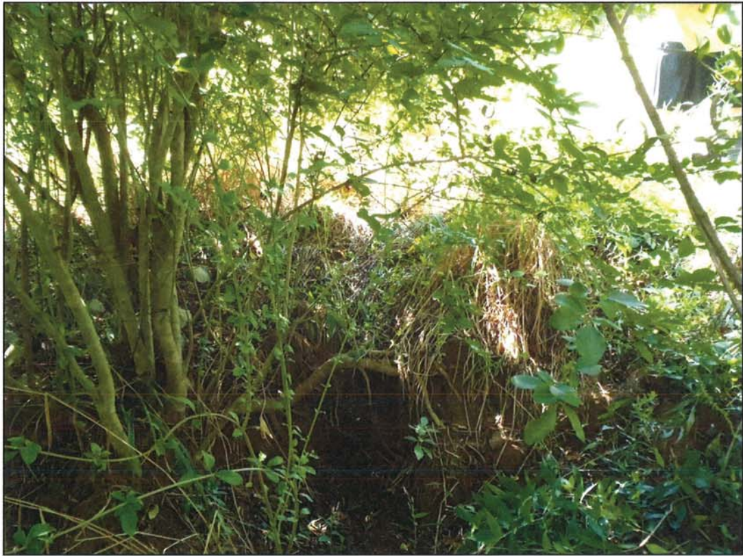
PHOTOGRAPH 35: RIP-RAP. WELTAND DRAINAGE.
