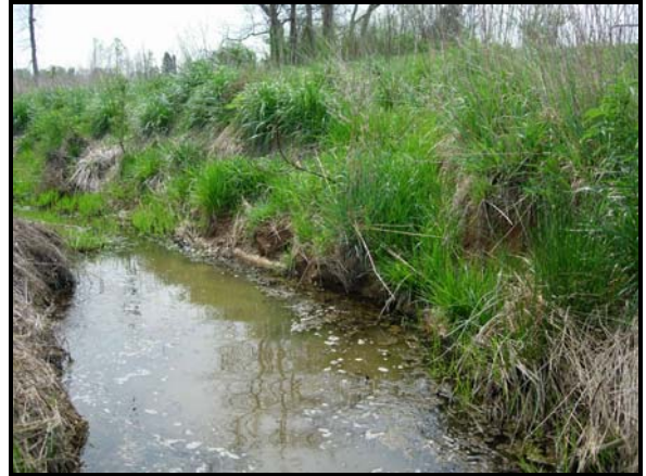
Toe Erosion along left bank (photo taken looking upstream)
