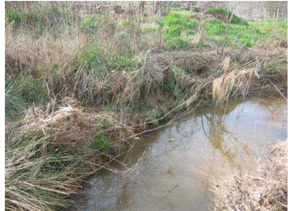
Photo 4. Bank Erosion (Station 19+15 along plan view)
