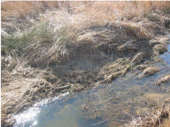
Photo 2: Bank Undercut/Erosion (Station 16+10 along plan view).
