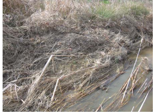
Photo 3. Bank Erosion (Station 16+10) upstream of J-hook
