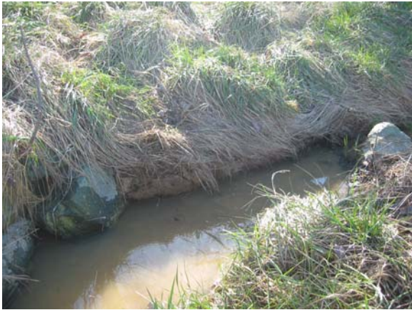
Photo 2: Bank Undercut/Erosion (Jan 31 - IMG 5278 – Pts 837) (Station XX along plan view).
