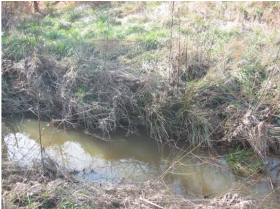
Photo 2: Bank Undercut/Erosion (Station 11+65 along plan view).
