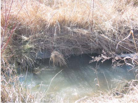
Photo 1: Bank Erosion (Station 17+55 along plan view).
