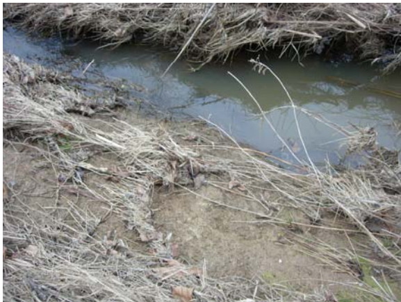
Photo 3. Representative bare bank problem area (Station No. 16+40; view across channel from left bank on 3-18-2008). Bare bank is on left bank (i.e., nearest in photo).
