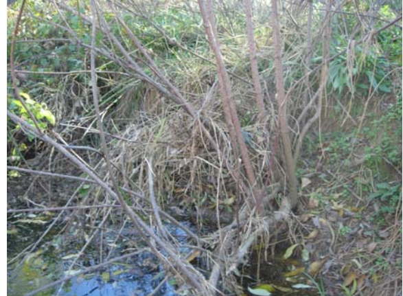
Photo 2: Representative bank erosion problem area (Station No. 19+30; view upstream, right bank; 11-6-2008).
