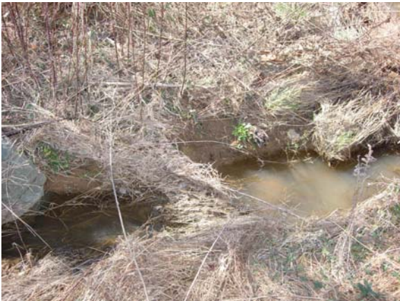
Photo 3: Representative bank erosion problem area (Station No. 10+78; facing left bank on 3-06-2008).
