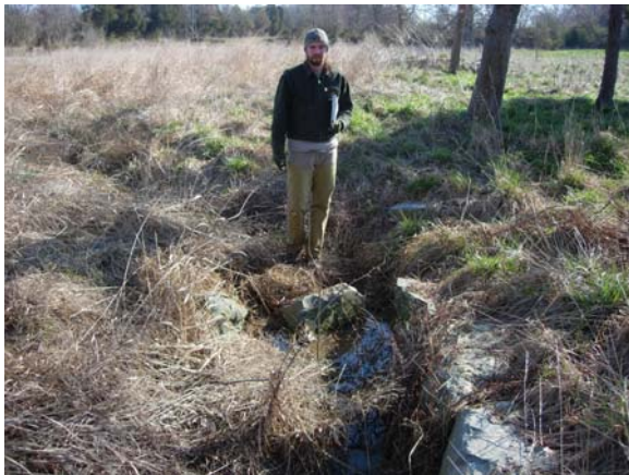
Photo 3: Representative problem J-hook (Station No. 14+92; view upstream; 2-28-2008).
