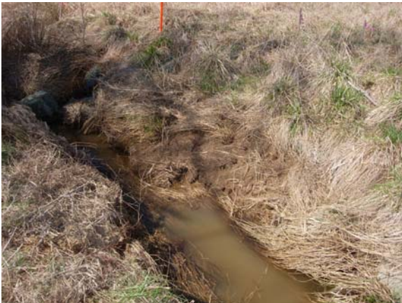
Photo 2: Representative bare bank problem area (Station No. 18+61 – 19+67; view upstream; 3-05-2008).
