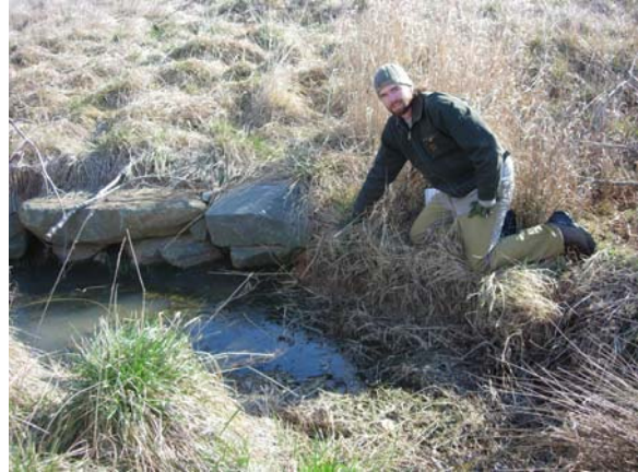
Photo 2: Representative bank erosion problem area (Station No. 18+26 – 18+31.5; view of left bank; 2-28-2008).
