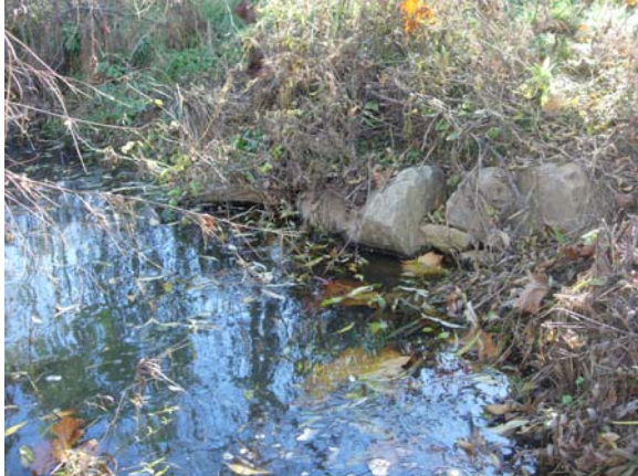
Photo 1: Representative jhook problem area (Station No. 19+45; view of right bank, downstream, 11-6-2008).
