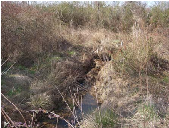
Photo 3: Representative multiflora rose ( Rosa multiflora ) problem area (Station No. 11+60; view downstream on 3-06-2008). Rose is located on left bank in upper left corner of photo.
