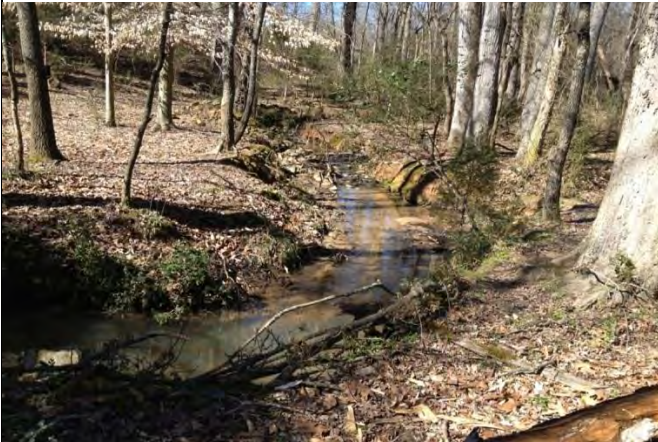
View looking upstream at minor stream bank erosion/channel incision (10/28/12)
