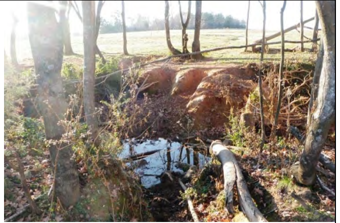
View looking at right stream bank erosion and channel incision (2/9/11)
