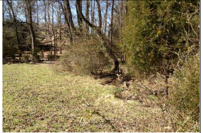
View looking downstream at left stream bank erosion and minimal buffer vegetation (2/20/13)
