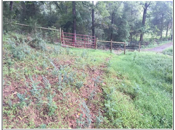
2) Vegetation Problem Area #2 – Right bank of Reach 4 near Station 53+50, Sept. 2016
