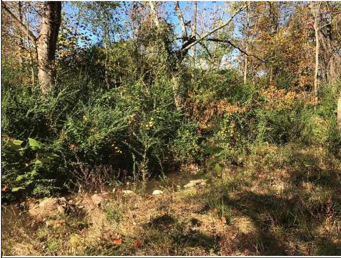
1) Vegetation Problem Area #1 – Right bank of Reach 5 near Station 28+50, October 2016
