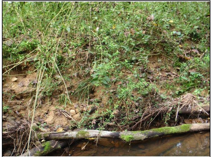
SPA: Bank scour along Reach R4 (~43+50)
