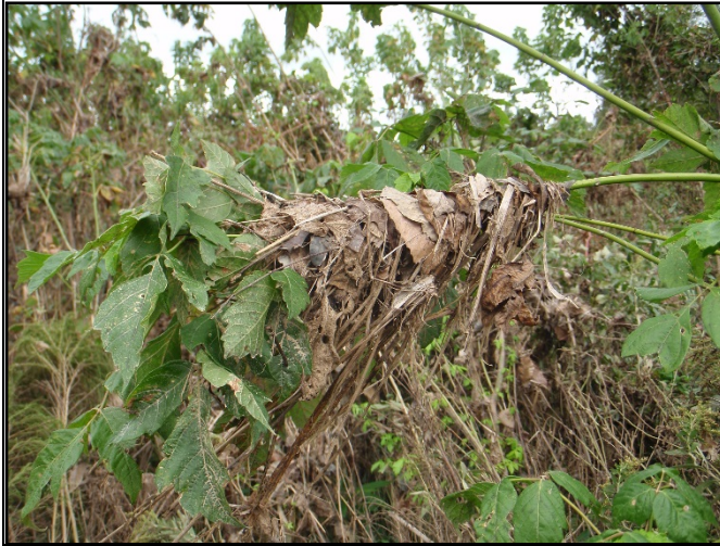
Reach R1: Debris caught in trees, Station ~18+00
