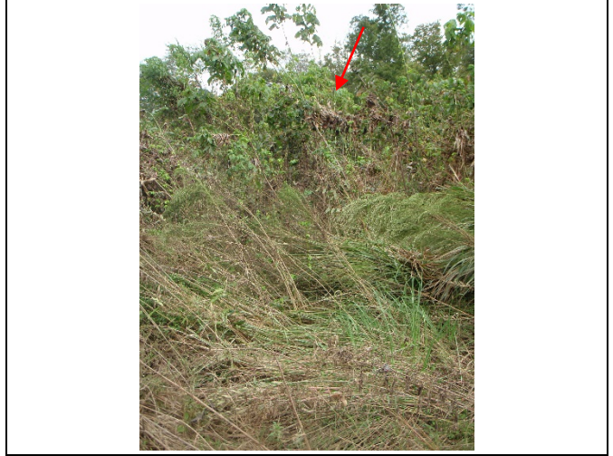
Reach R1: That same debris as observed from the stream at Station ~18+00
