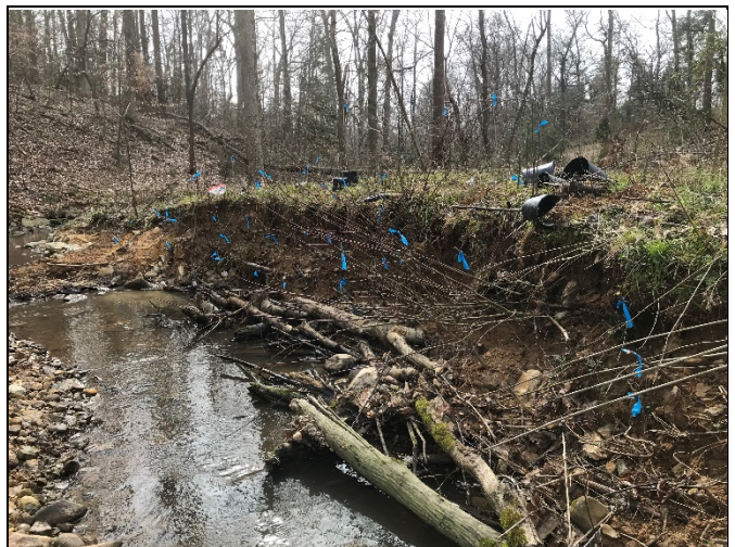
Reach R4 Station 43+50: Bank repair with livestock and 1-gal plantings into stream bank (Feb 2019)
