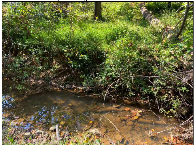
Reach R4 Station 43+50: Stabilizing and vegetating from previously documented bank scour from Hurricane Florence in Sept 2018 (photo from Oct 2020)
