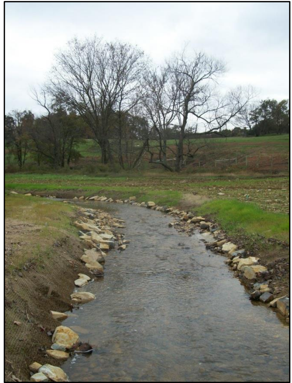
PID 19: Station 25+90 – Downstream (11/5/15)
