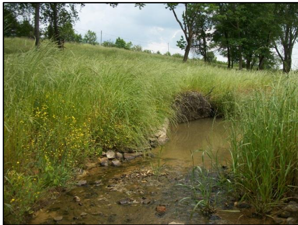
PID 10: Station 18+10 – Downstream (5/11/16)
