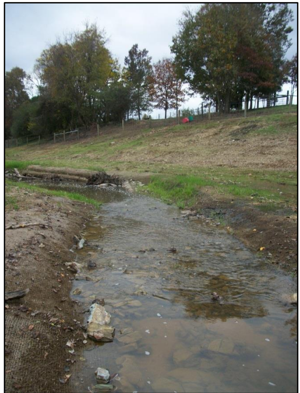
PID 8: Station 16+25 – Downstream (11/5/15)
