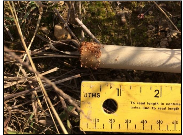
Crest Gauge Photo 2 (11/03/16)
