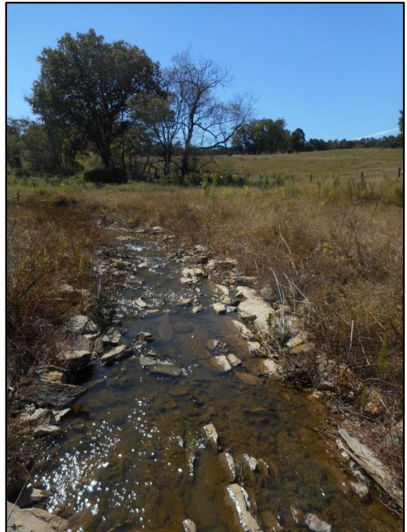
PID 19: Station 25+90– Downstream (10/11/16)
