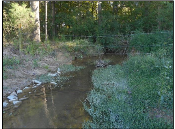
PID 41: Station 48+60 – Downstream (10/11/16)
