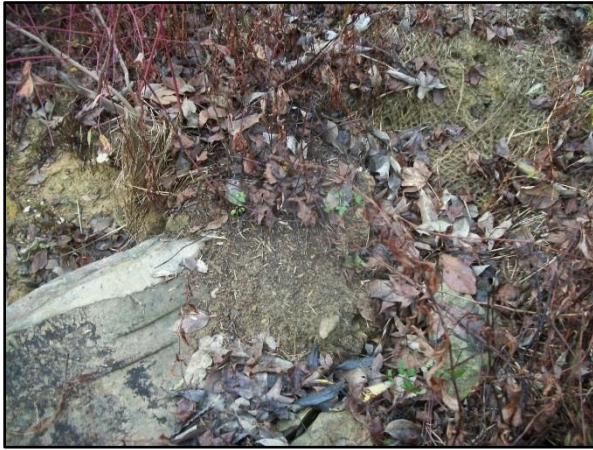
SPA2-1 – Station 16+20 - Erosion around right seal of boulder step. (11/09/17)
