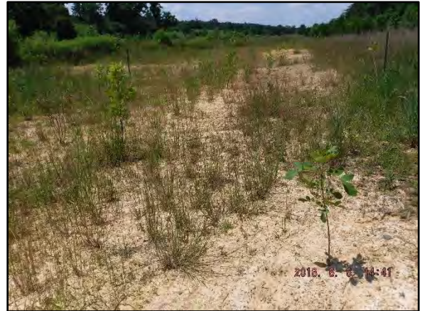
VPA 3-7 – Station 48+60 – Upstream photo of bare areas, areas of poor growth rates, and areas where supplemental plantings were installed. (06/06/18)
