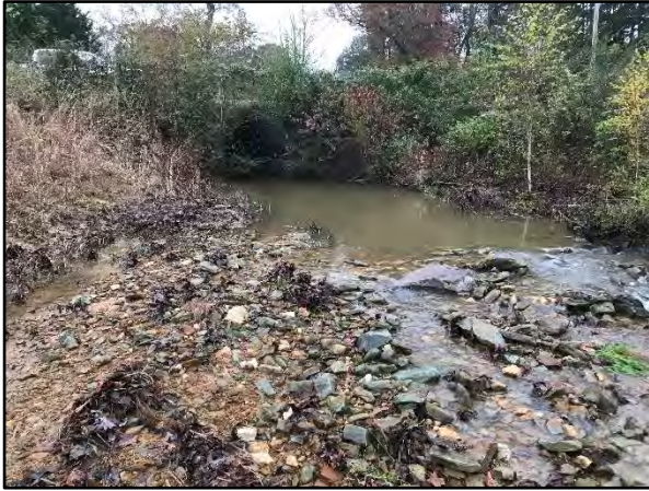
SPA 3-1 - Station 10+10 – Stream banks downstream of culvert have eroded and washed away during flooding in 2018 (11/14/18)
