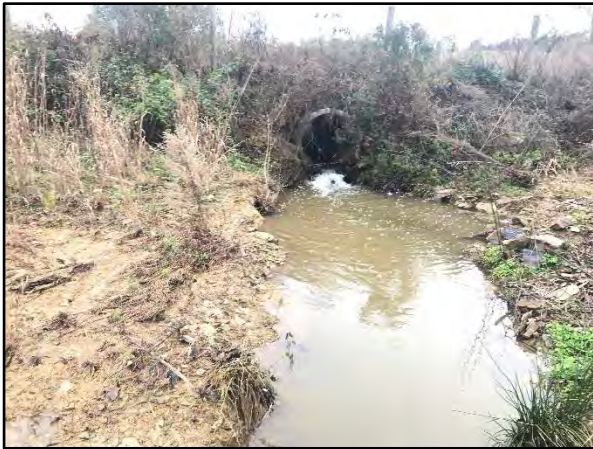
SPA 3-2 - Station 20+50 – Stream banks downstream of culvert have eroded and washed away during flooding in 2018 (11/14/18)
