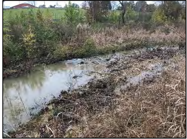
SPA 3-1 - Station 10+10 – Stream banks downstream of culvert have eroded and washed away during flooding in 2018 (11/14/18)
