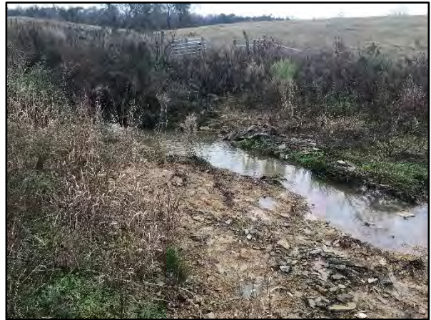
SPA 3-2 - Station 20+50 – Stream banks downstream of culvert have eroded and washed away during flooding in 2018 (11/14/18)
